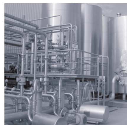
> Cleaning-in-place systems at a dairy factory.
